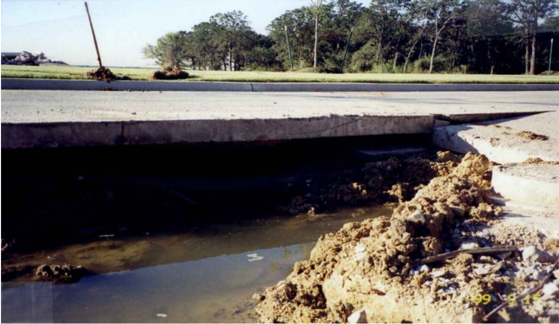
Photograph 2. Gross settlement of utility backfill around a sanitary sewer manhole.
