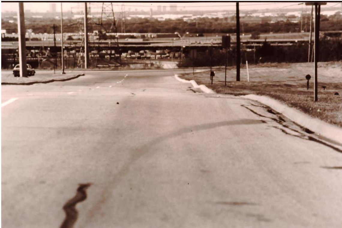
Photograph 3. Differential heave along Northgate Boulevard, Irving, Texas. Pavement is approximately 25 years old.
