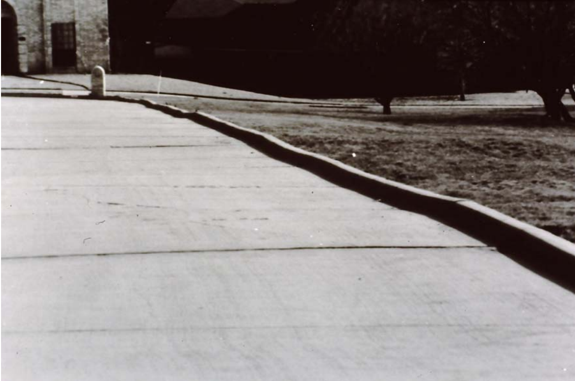
Photograph 4. Differential heave of subdivision pavement in Carrollton, Texas. Pavement was approximately 2 years old.
