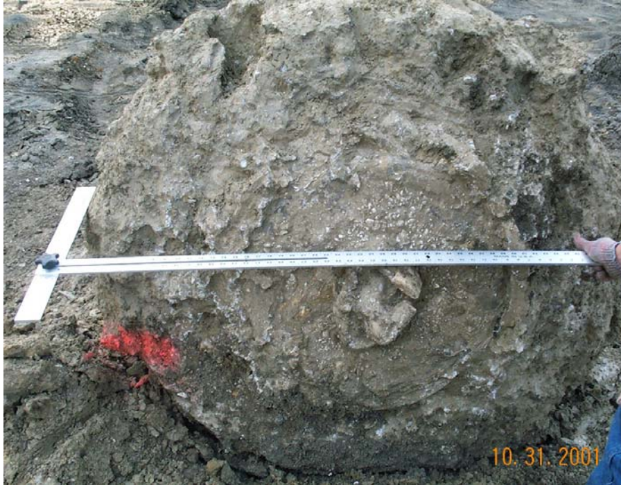
Photograph 1. Bottom of exhumed pier. Note how poorly the underream was cleaned of debris at time of concrete placement.
