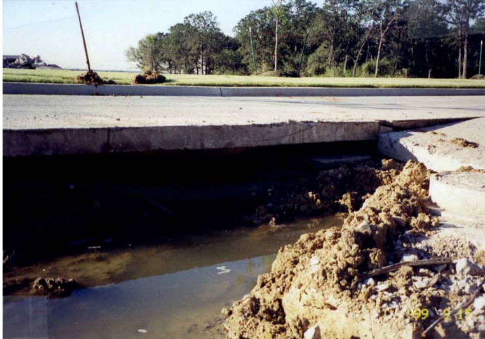
Photograph 2. Example of degree of utility line excavation settlement.
