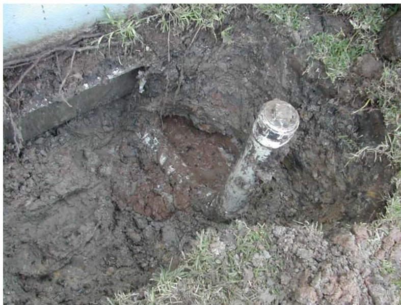
Photo 1: Water Bearing Trench Backfill
