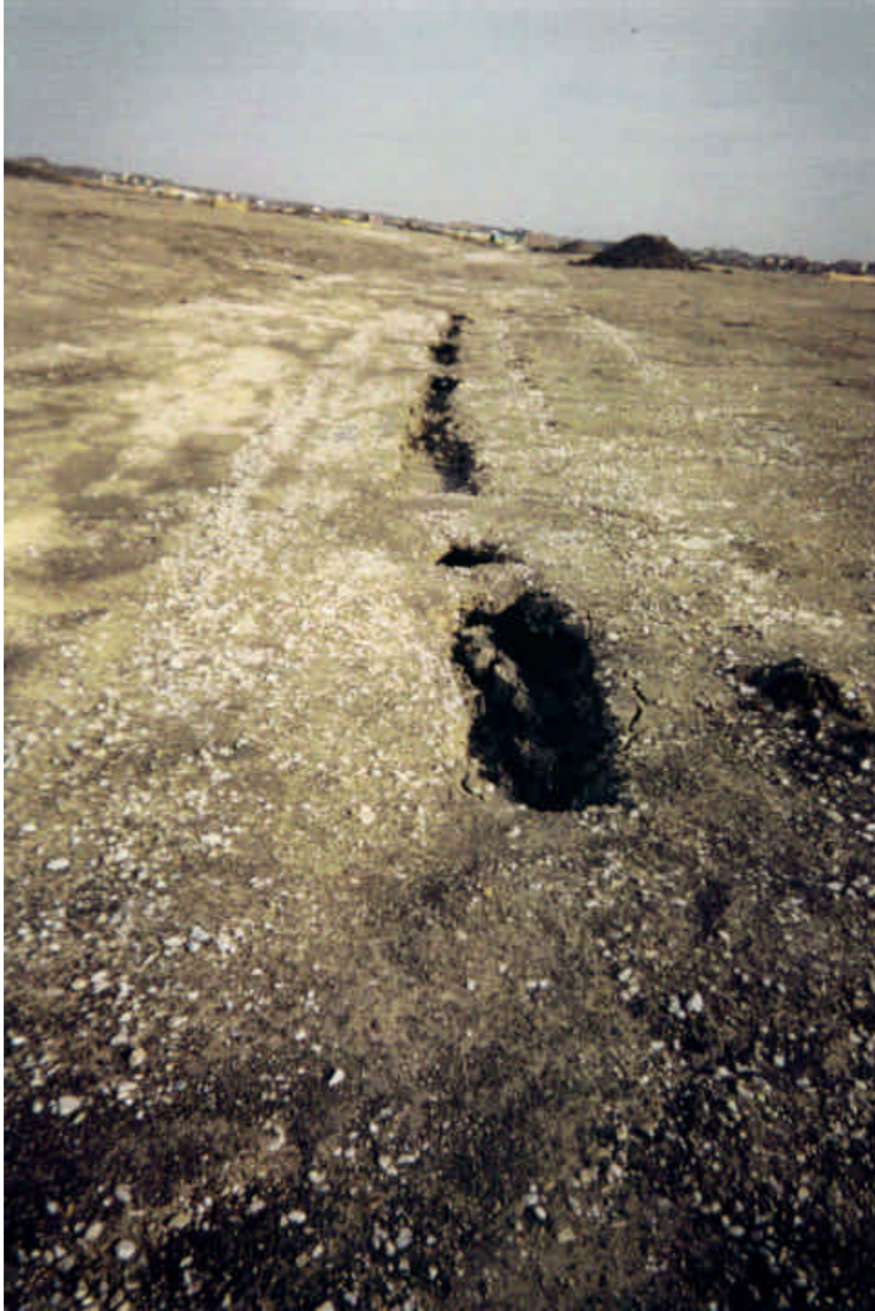
Fig. 4 Post construction settlement of utility trench backfill.
