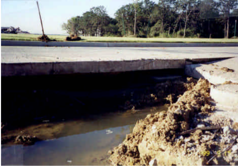
Fig. 5 Post construction settlement of utility trench backfill. Note the resulting void beneath the pavement section.
