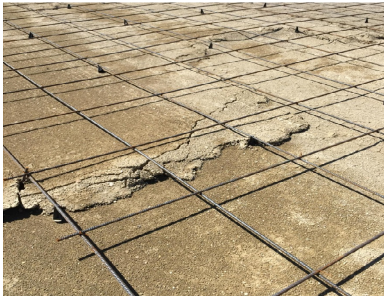
Figure 3. Close-up of shear failure. Note iPhone below reinforcing at left for relative size.
