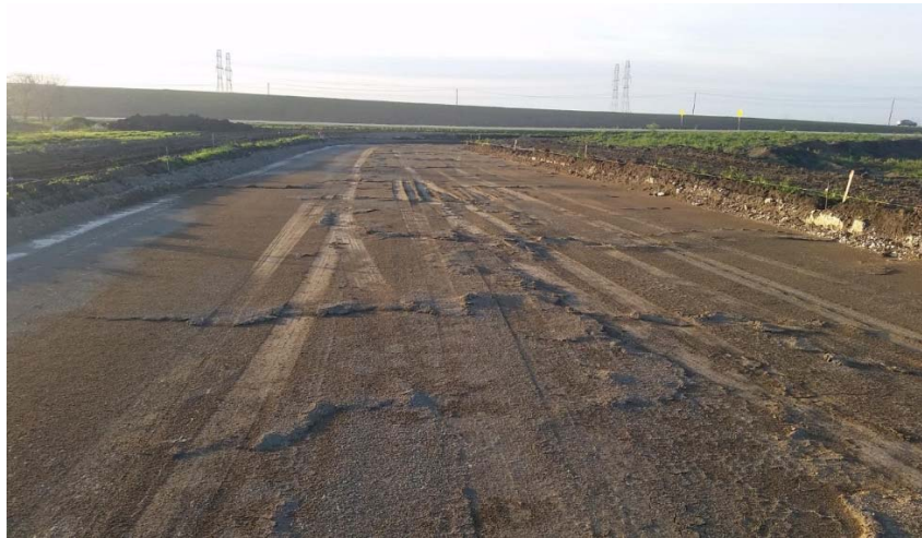
Figure 2. Photo of general failed condition, Challenger Drive.
